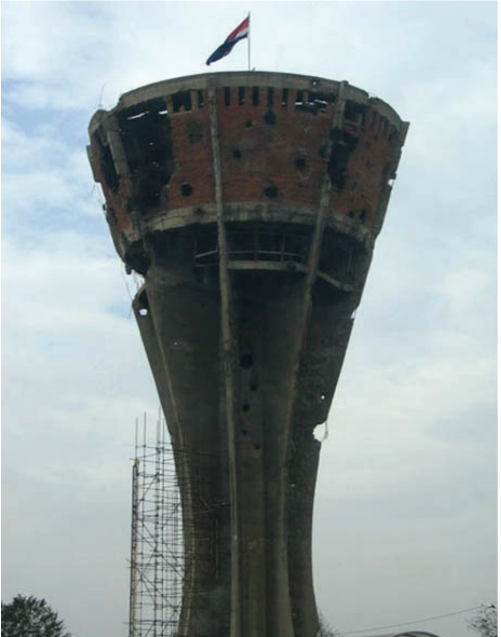
Water tower, Vukovar (photographs taken from the archive of the Croatian Military Journal)
