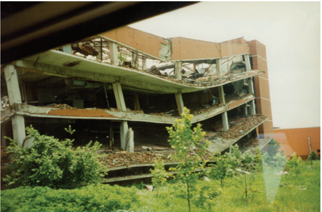
Remains of the building "Borovo-Commerce" in Borovo Naselje, destroyed in the last attacks by the JNA on November 18 th and 19 th , 1991; the photograph was taken after Vukovar was occupied by Serbs (photograph taken by: Božo Biškupić)
